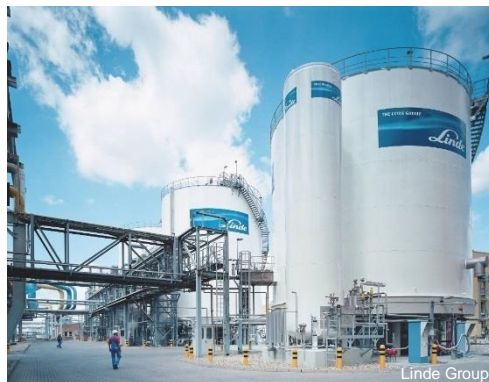
liquid gas storages with vacuum super insulation
