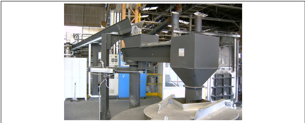
Fig. 4: Induction furnace with chip conveyor
